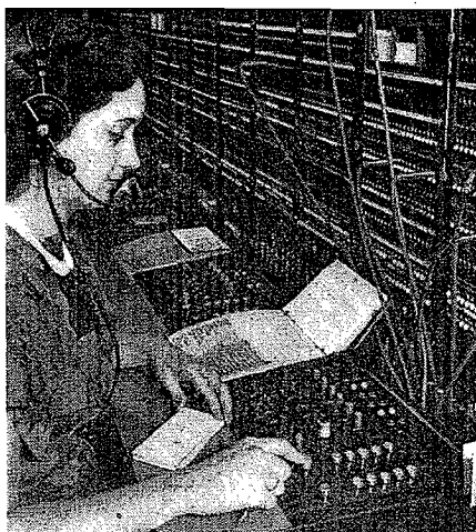
Figure 2. Outward operator at toll switchboard
